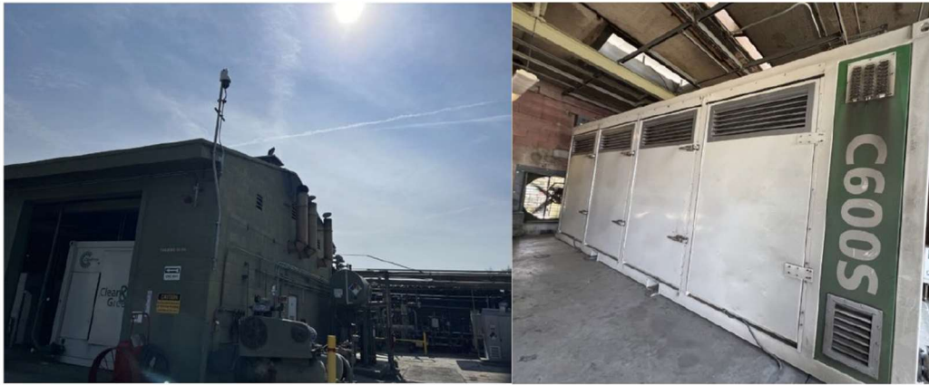
Figure 9: Outside and inside of the turbine room with C600S Capstone microturbine. Clean and well maintained. Fully registered and permitted to operate per AQMD. Good maintenance records.
